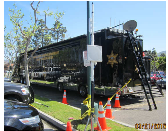
2.4-GHz Ubiquiti NanoStation and 5-GHz Ubiquiti Rocket with dual-channel flat-panel antenna at OCSD's Samantha I receiving video streams from two strings of ipCams.
